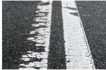
Figure 5: Faded road markings.
