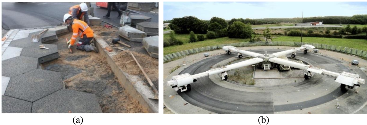
Figure 4: (a) Construction of the test structure at Gustave Eiffel University, (b) Fatigue Carousel (Gustave Eiffel University – Nantes, France).
