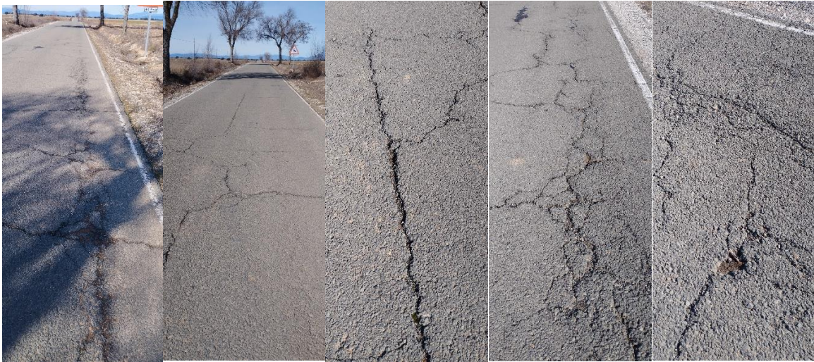
Figure 12: Surface defects in CM-2008
