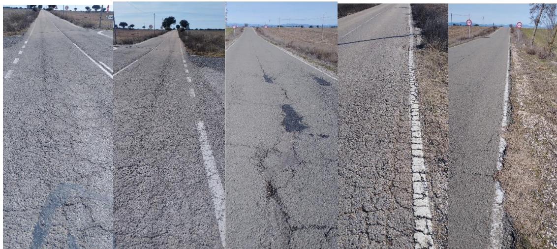
Figure 13: Surface defects in CM-1000
