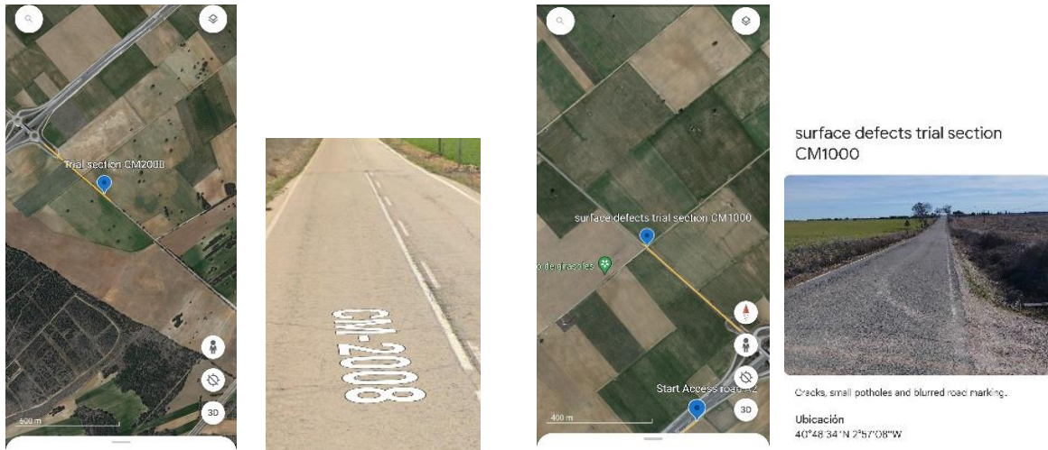
Figure 6: Location and coordinates for the evaluation of the surface defects in CM-2008 and CM-1000
