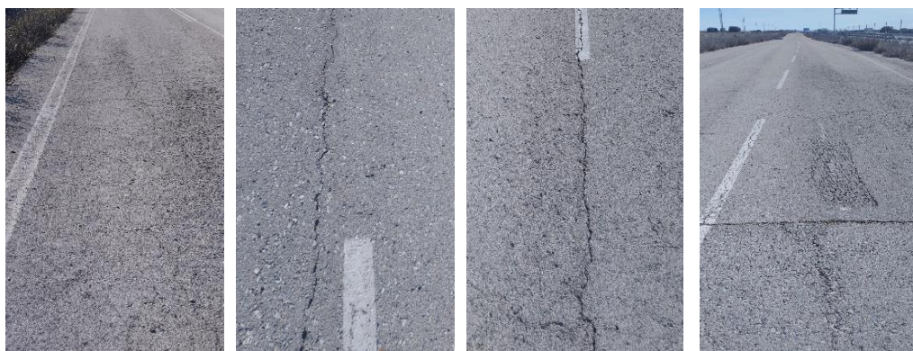
Figure 8: Cracks and road markings blurred in the section selected in the old N-2
